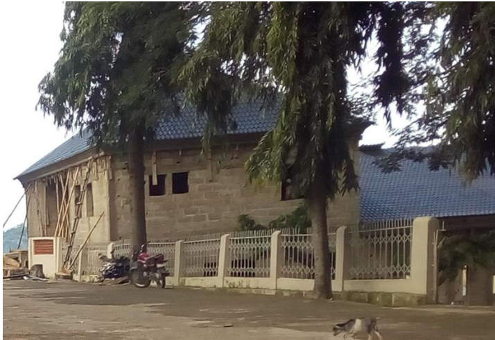
Pix 9: An image of the On-going construction of the 3,500-capacity Town Hall Source: Fieldwork, 2019
