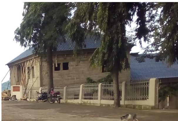
Pix 9: An image of the On-going construction of the 3,500-capacity Town Hall
